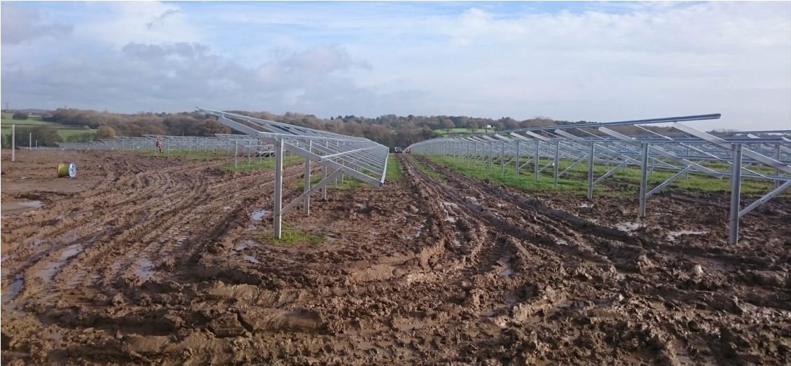
Inserts 36 and 37: Winter Installation (2015) and Operational Site (2022)
